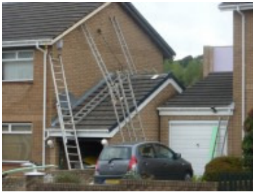
Falls risk during soffit replacement work
